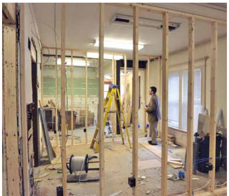
Greg Kovacs, executive director, checks the progress of renovations at The Samaritan Counseling Center's new home at 1612 Genesee Street in Utica.
